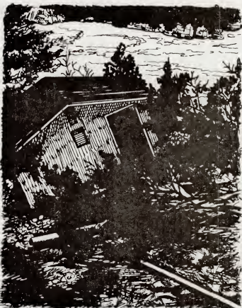
Treatment plant housing sits a tilt off its foundation after flood near Kerr Dam last June.
